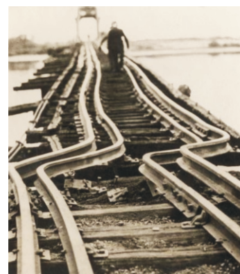
Figure 12.5: Railroad tracks that have expanded due to heat on the Delaware river (1935).
